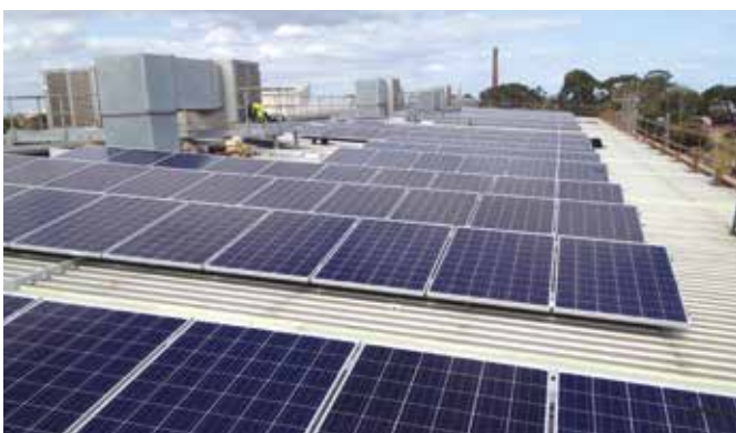
99.7 kilowatt Photovoltaic system on the main rail workshop at the Newport, Victoria, comprising of 60 solar panels.
