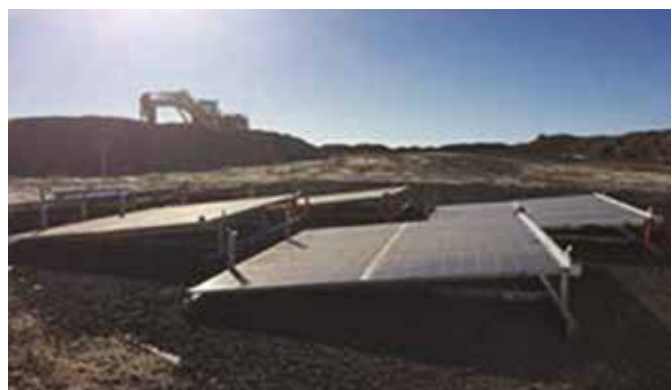
Solar panels at Commodore Mine crib hut.
