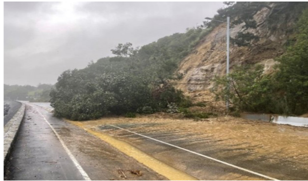
Figure 4: Emergency road closure on Tāmaki Drive in Auckland Jan 2023 – a high impact road with 30k VPD – opened one-way within 48 hours.
